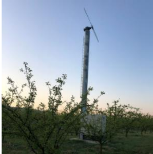
Figure 12 Fixed Antifreeze Tower
